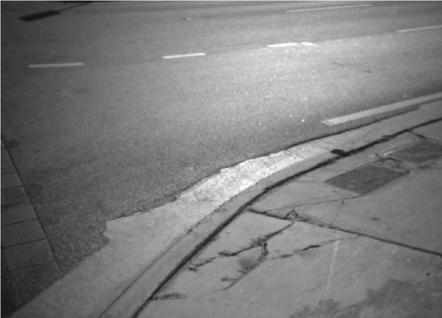
Figure 9. Possible Damage on the Curb from Bus U-Turns
